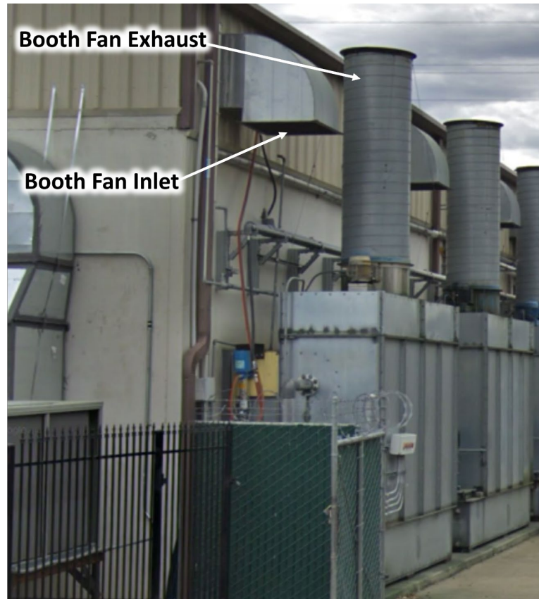
Figure 11. Booth Ventilation Exhaust System. (Source: Google Street View, annotations by CSB)
